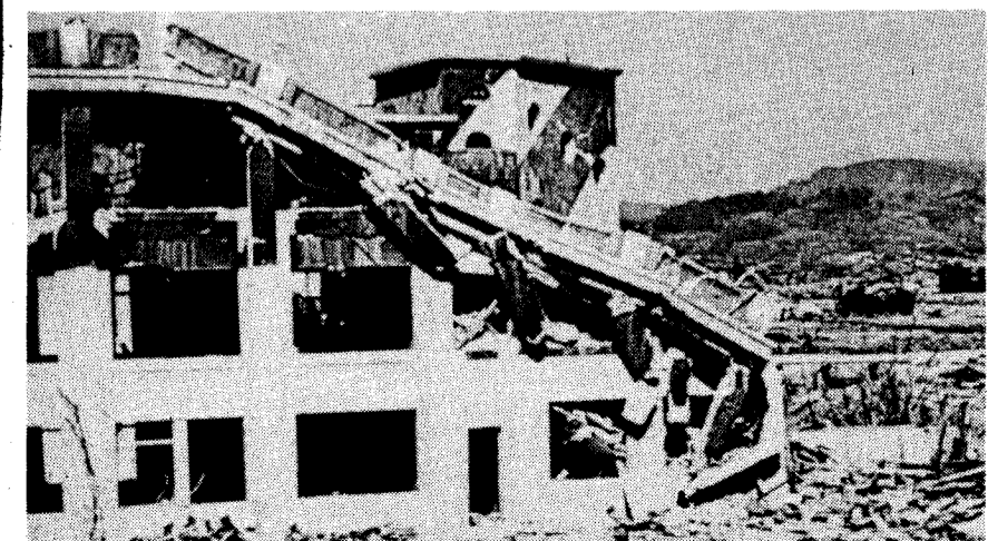
School building in Nagasaki where 133 out of 152 children died — people in Europe are more and more determined it will not happen again
